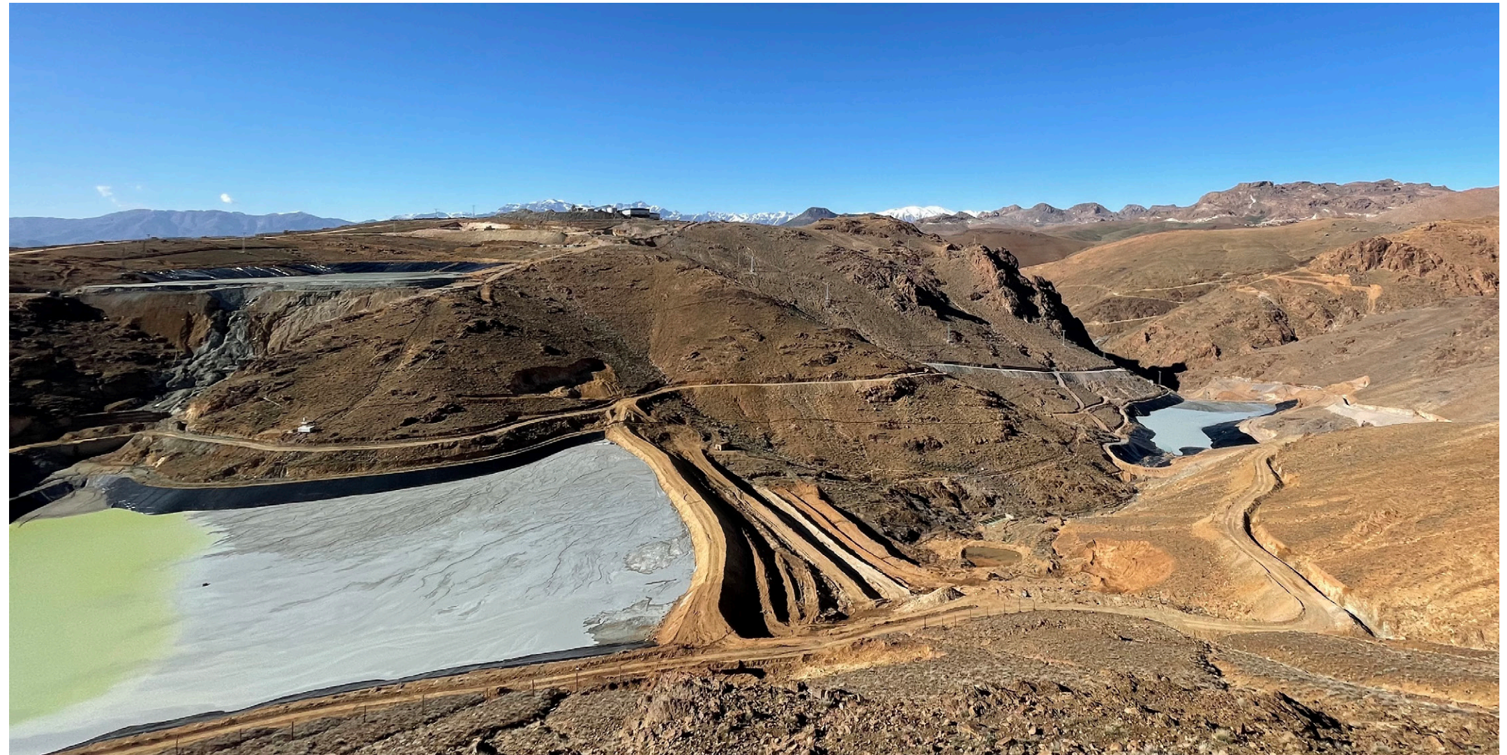
Left: TSF #3 (cyanide circuit) in the center. TSF #2 can be seen in the background on left, above TSF #3, and TSF #4 on the right side, downstream from TSF #3.
