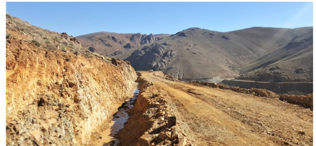
Below: The storm water canals and service roads run on both sides of the valley.
